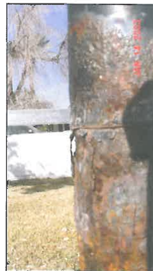
Photo 4b. Layers of Rust, Pushed Away From Pole Metal At The Joint Between The Lower And Middle Sections Of The Pole
