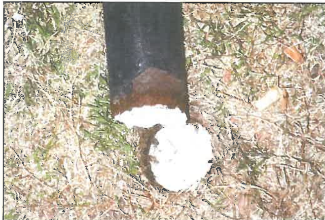
Photo 1d [2] . Close-up Of Broken Pole, At The Break.
