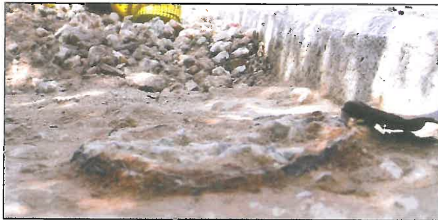
Photo 7b. Close-up Of Corroded Pole Stub In Desert Landscaping
