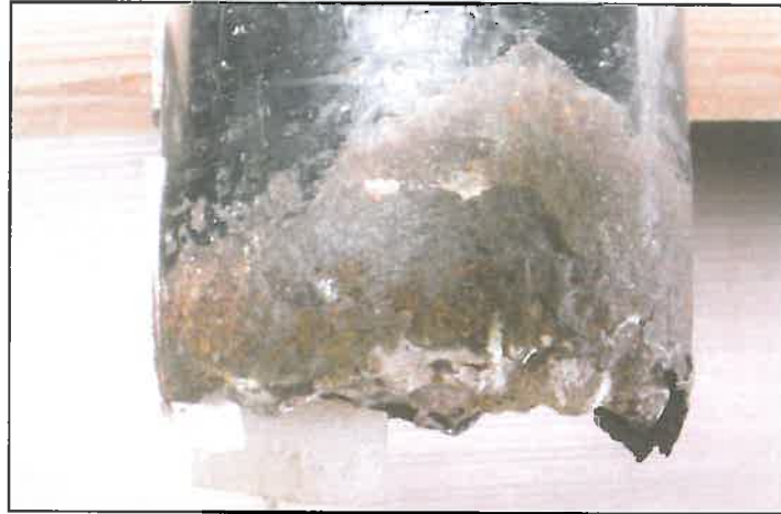
Photo 2. Close-up View Of Subject Pole End, Showing Corrosion.
